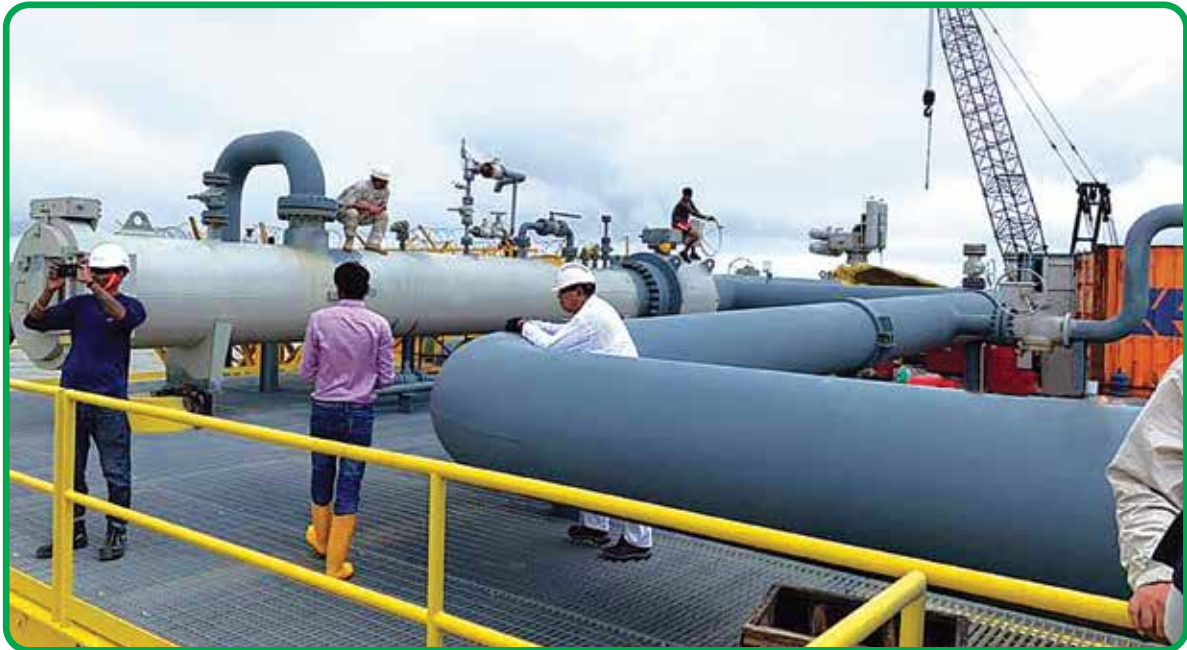
Construction of platform and piping facilities at Zero Point under Maheshkhali Zero Point-CTMS pipeline project
