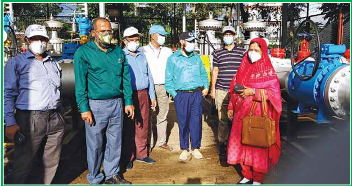
Site visit for conducting feasibility study of proposed Dhanua-Mymensingh Gas Transmission Pipeline
