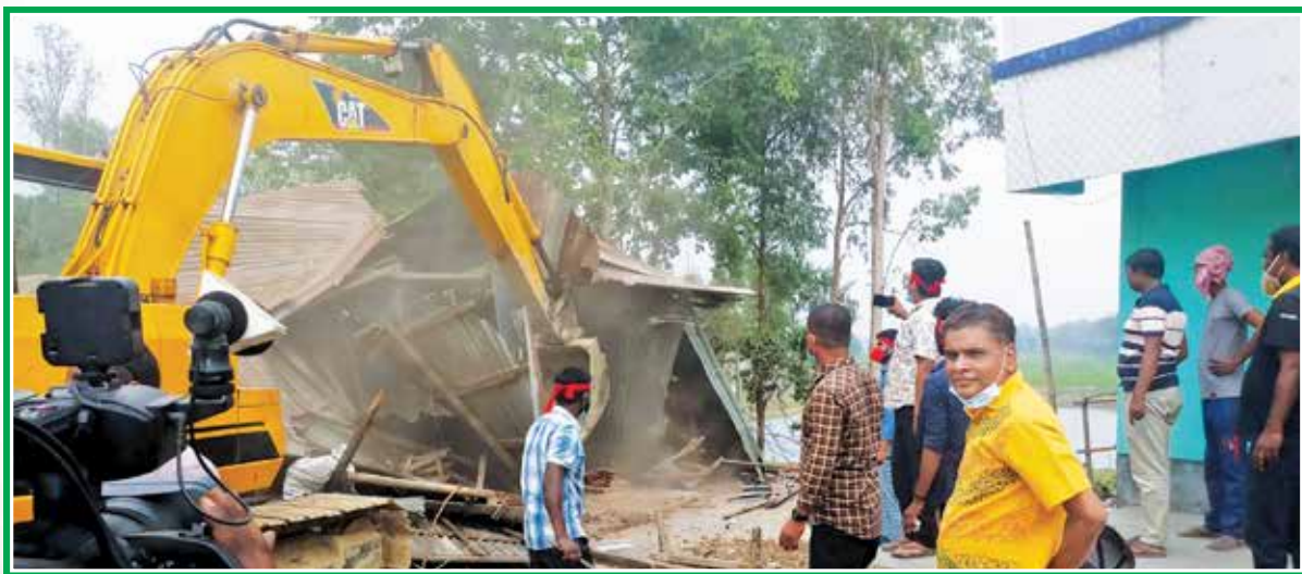
Eviction of illegal structure over pipelines by GTCL
