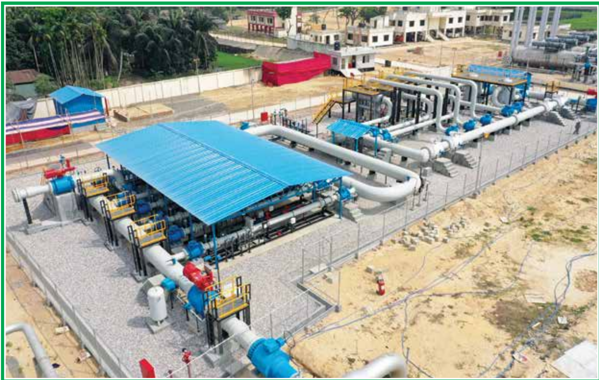
1500 mmscfd capacity metering station at Maheshkhal under Maheshkhal Zero point Project
